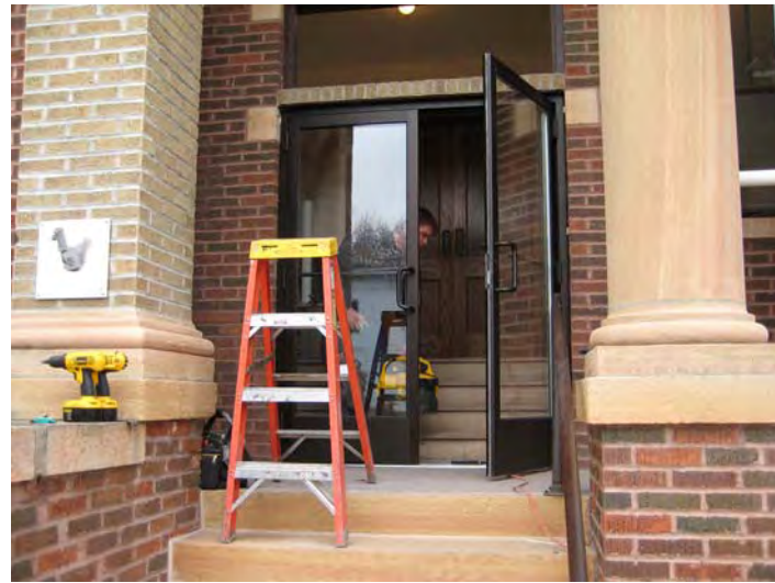
Pictured above: Waseca Glass workmen install the new front doors of the Museum in October.
